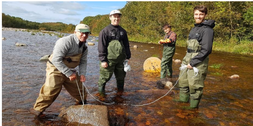
Figure 6. Installation of fibreoptic DTS cable as part of trial involving Dr. Kurylyk's research group, October 2019.
