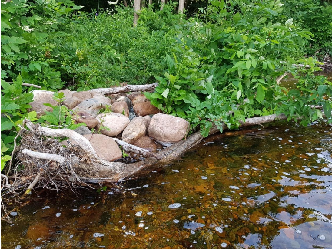
Figure 3b-1. Deflector in western split installed summer 2020 to prevent an imminent breach
