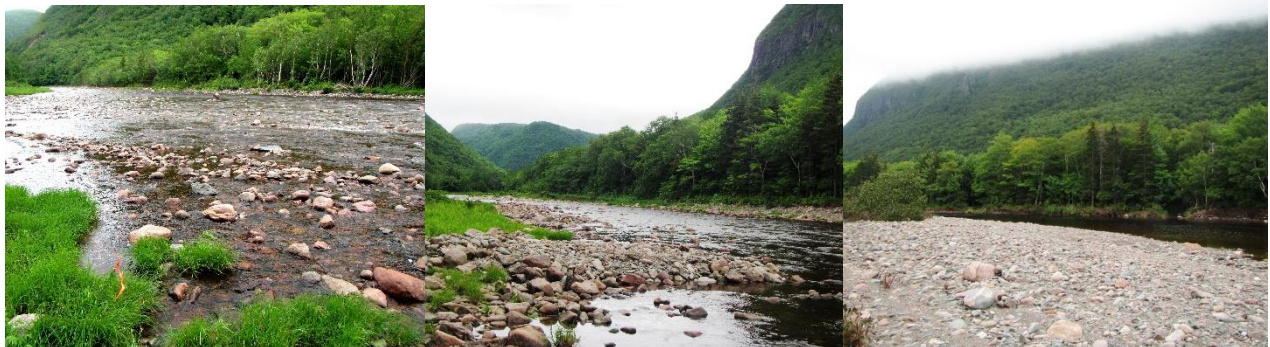
Sample project photos from downstream start of Below Fence Pool work site in 2015 showing view looking upstream from right bank just before work started (left), after rock retarding bars were installed (middle), and the changes to the site following major flood event in August 2015 (right).
