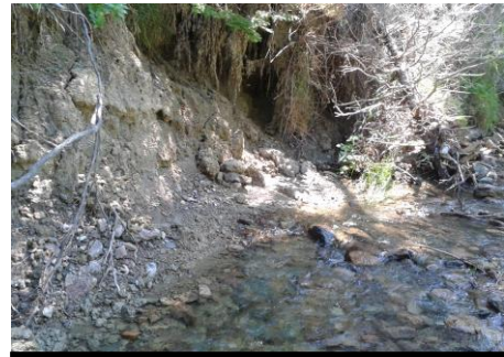
9a – Example of erosion on right bank
