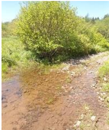
6a – Brook flooding road at bridge
