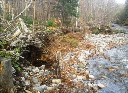
9a – Unstable, eroding left bank at upper limit
