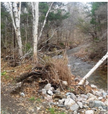
9b – Erosion of bank and road on left bank just downstream from bridge
